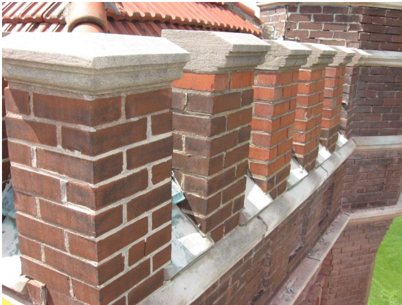
Figure 16. Battlement on west elevation. Note lighter colored bricks indicative of previous repairs.
