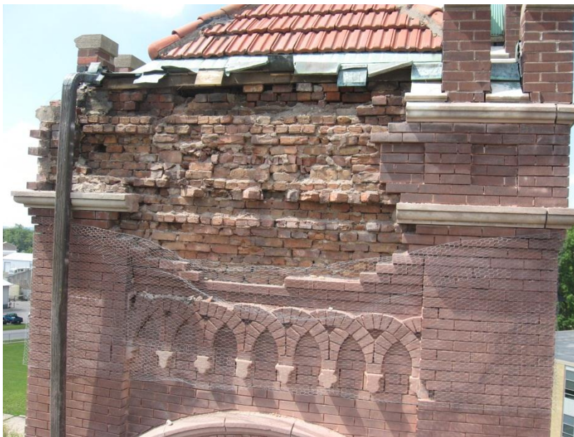
Figure 6. Overall view of collapsed portion of bell tower, north elevation.
