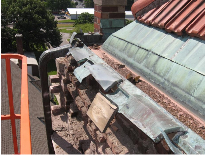
Figure 11. Copper gutter and flashing on north elevation.
