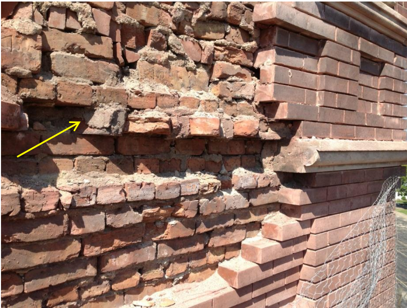
Figure 10. Note no evidence of metal ties in backup brick. Course of diagonal header bricks shown by arrow.
