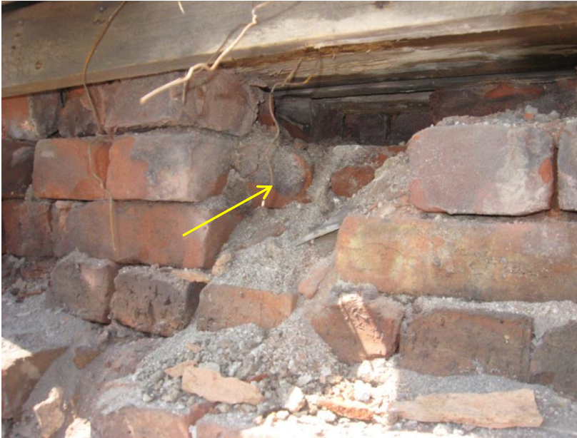
Figure 9. Backup brick masonry loose and easily removed by hand (arrow).
