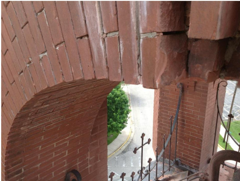
Figure 29. Dislodged bricks in the large arch, east elevation of bell tower.
