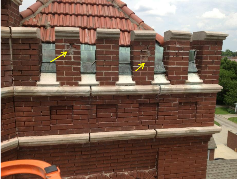
Figure 25. South elevation battlement. Note some loose pieces of masonry had been removed (arrows).
