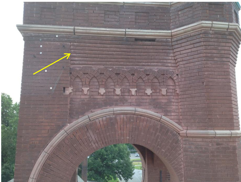
Figure 14. Overall view of west elevation of bell tower. Joints in stepped out portion of brick masonry (arrow) were ground out. Note missing bricks under limestone water table.
