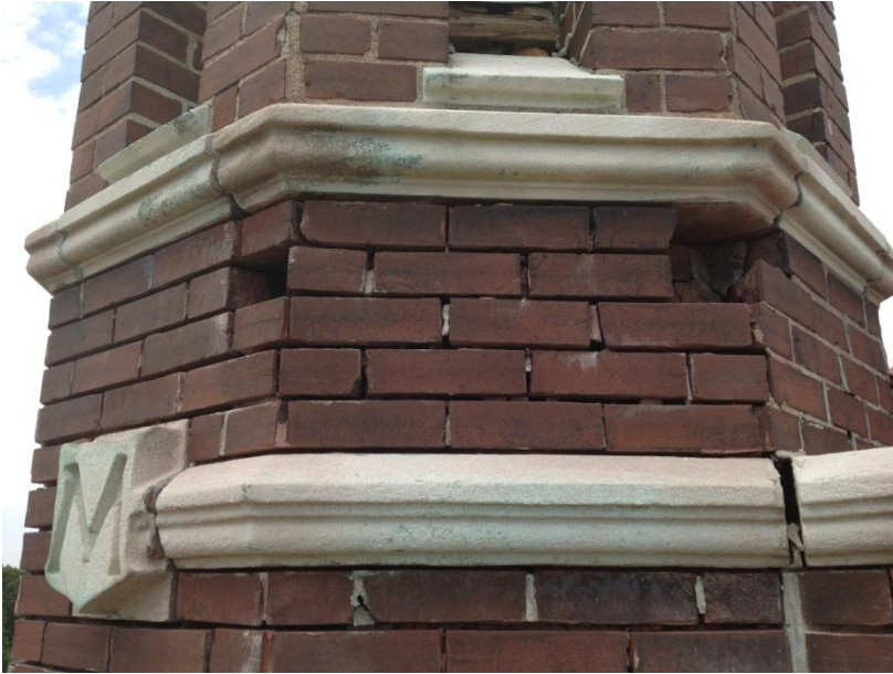
Figure 23. Removed face brick on turret below steeple. Backup brick also was loose and unsound at these locations.
