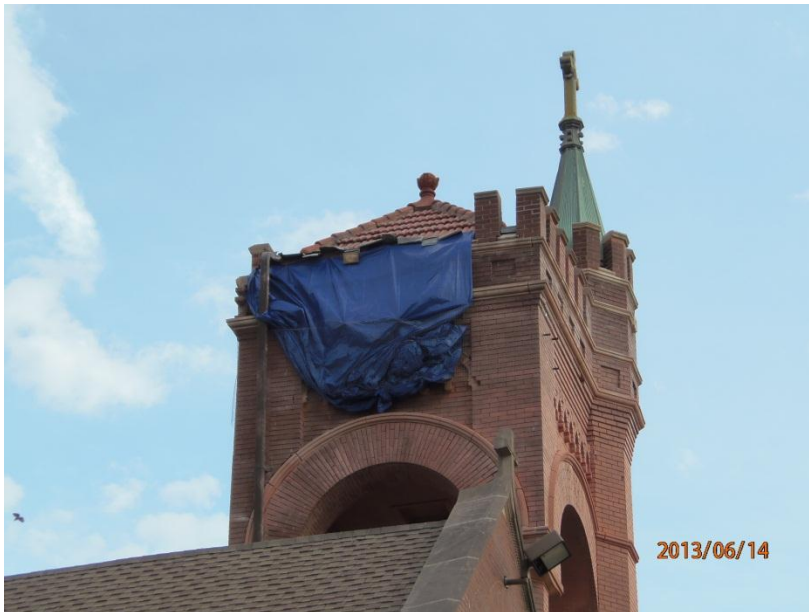
Figure 5. Tarps on north elevation of bell tower (photo by Catholic Mutual Group).
