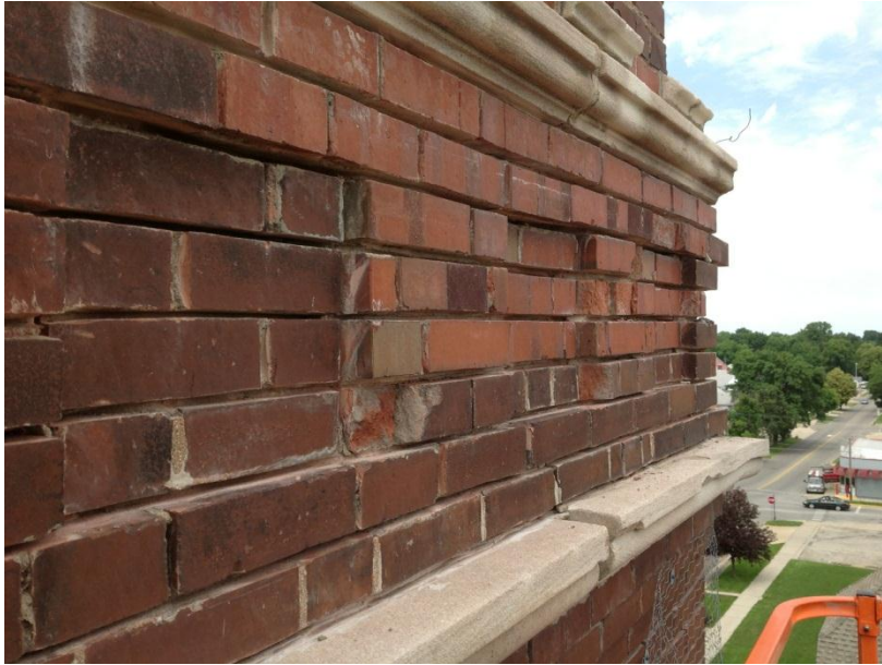
Figure 27. Partially rebuilt portion of facade above water table on east elevation of bell tower.
