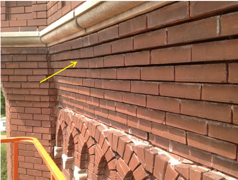
Figure 24. Stepped out portion of face brick on south elevation. Note deflection at loose brick (arrow).
