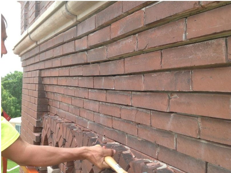
Figure 28. Waviness in bed joints at stepped out portion of face brick on east elevation.
