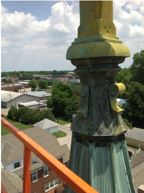
Figure 19. Base of cross at steeple. Overlap of copper sheeting allows some movement at this location.
