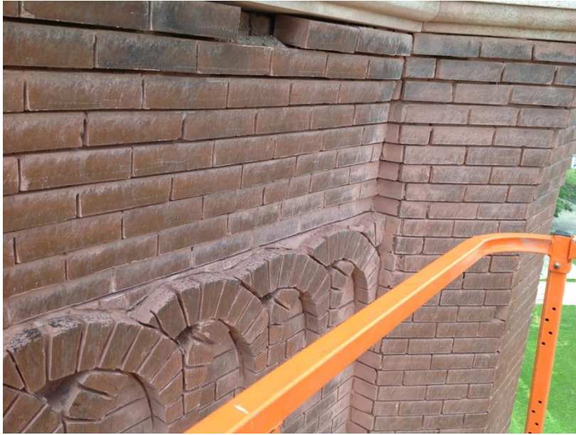
Figure 15. Close up view of stepped out portion of masonry showing profile and removed brick.
